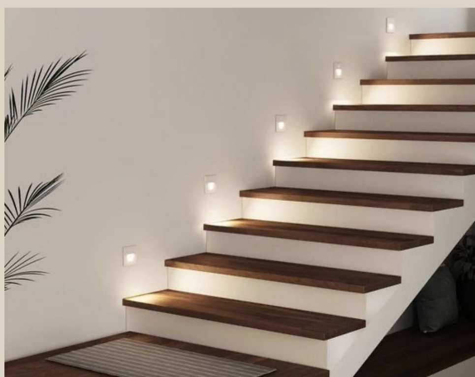
35. ESC01 ALPIN LED luminaire power MAX 8W color urban grey with 3000K warm light, recessed in stair walls
