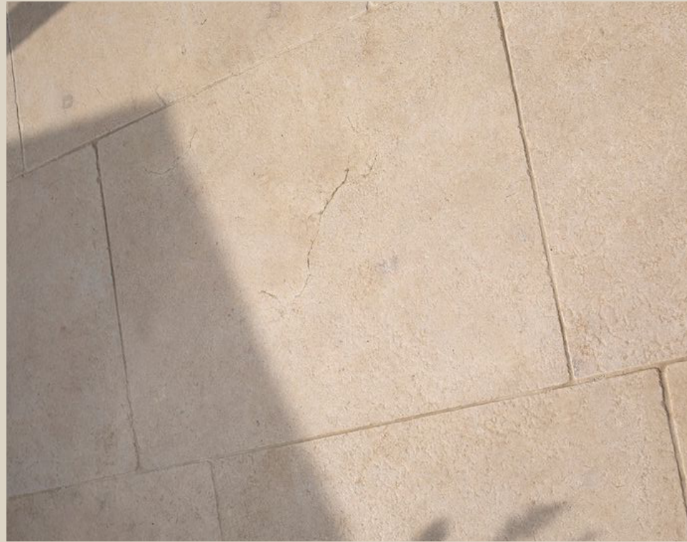
2. Floor finish For exteriors: Non-slippery light travertine marble, format: 40 cm x free lengths 2.02
